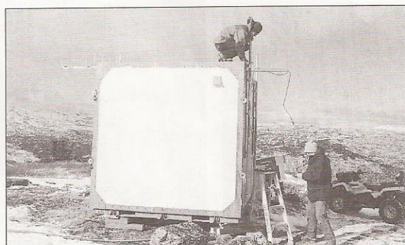
YARA installs a new repeater on Haeckel Hill.
